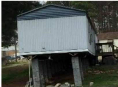
Figure 2.2. Ineligible dry-stack foundation
