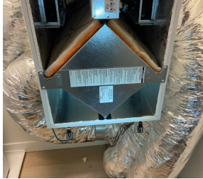
Northside Passive Air Source Heat Pump COP 3.3@47, 2.3@17
