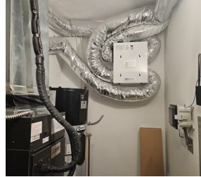
Hillcrest Village Air Source Heat Pump 19 SEER, 10.2 HSPF
