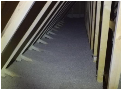
Don't provide photo that only shows ceiling insulation.
