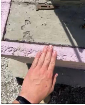
Don't measure insulation thickness without a measuring tape.
