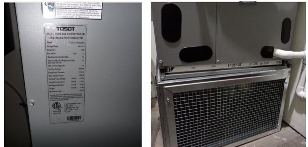
Do provide photo of mechanical equipment nameplate and filter.
