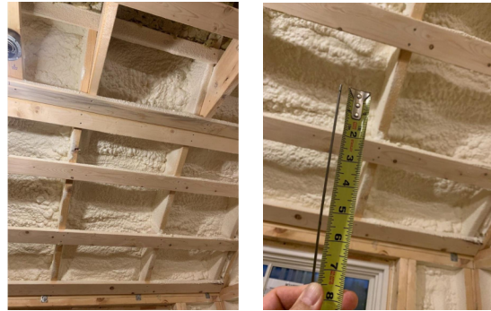
Do provide photo that shows spray applied insulation and measured insulation thickness.
