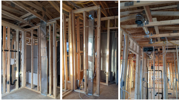
Don't simply provide photo of mechanical ductwork.
