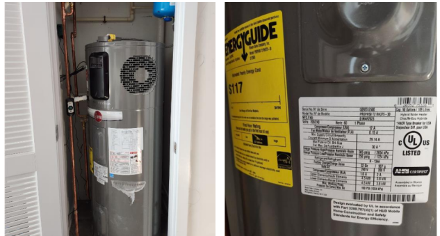
Do take close photo of DHW system nameplate and EnergyGuide label.
