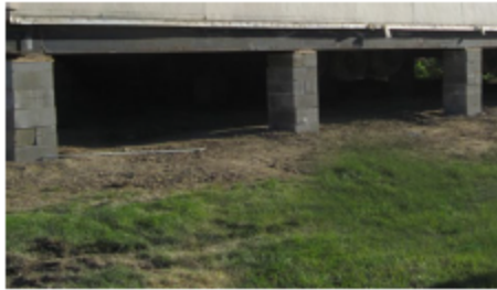
Figure 2.1. Ineligible dry-stack foundation
