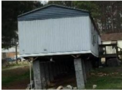
Figure 2.2. Ineligible dry-stack foundation
