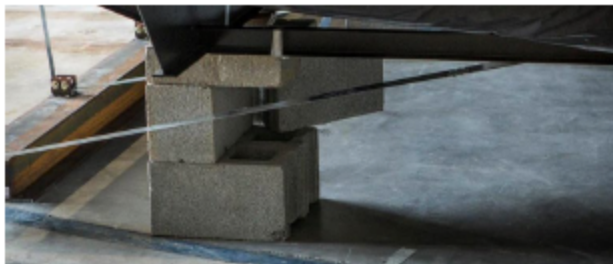
Figure 2.3. Ineligible dry-stack foundation
