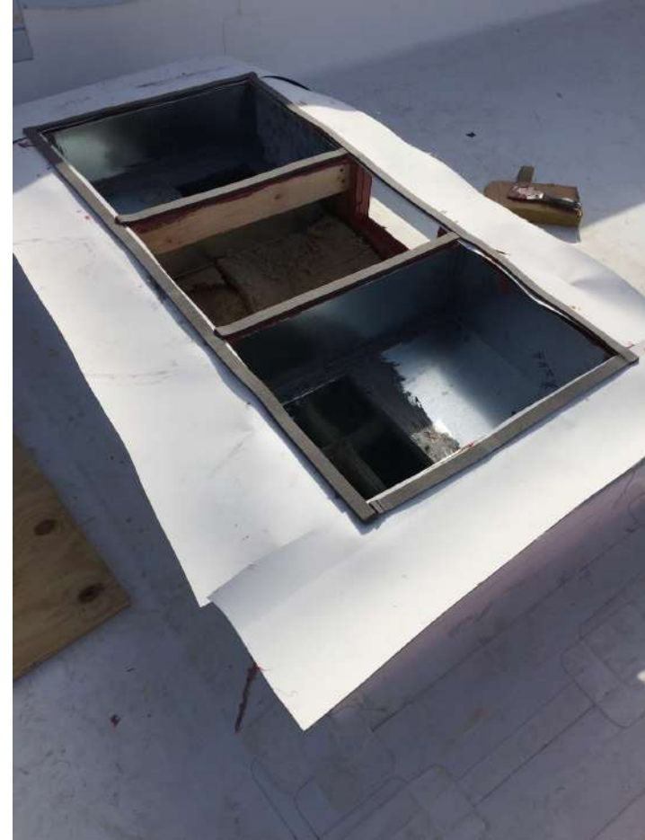
Roof: Curb for ERVs
