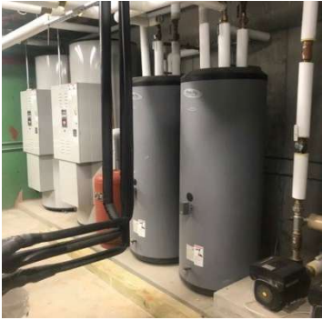
The Battery, PHIUS + Certified, 2017, DHW tanks for 25 units
