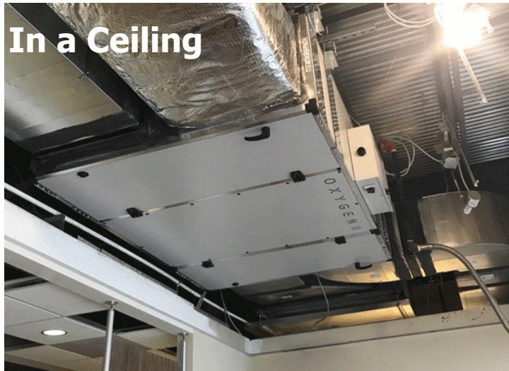
In a Mechanical Room
