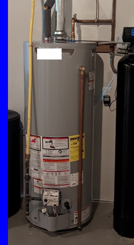
Hot Water Generation
